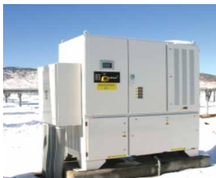
Source: Advanced Energy
